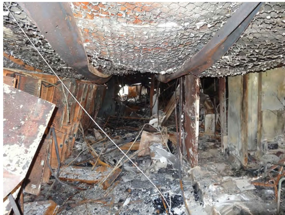
Figure 2. Interior of Burned Northeast Section of West Intermediate School (Source: ABS Consulting 2015).
